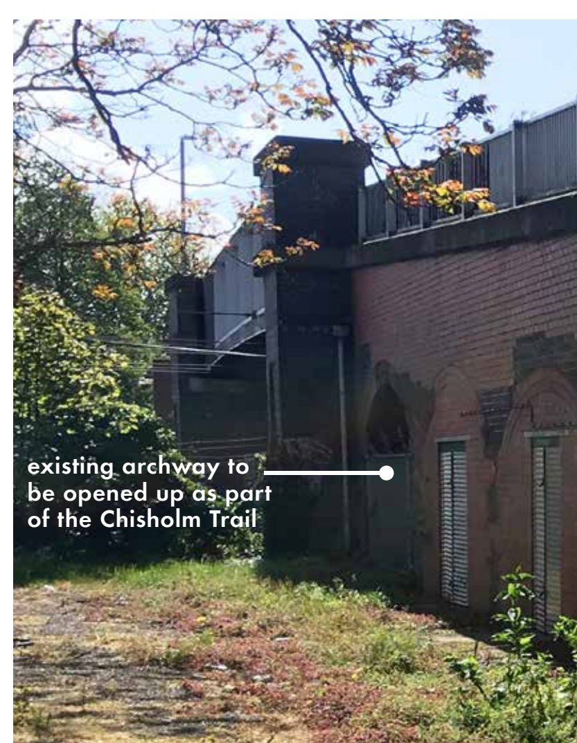
As part of the Chisholm Trail, the existing archway is to form a new cycle/pedestrian route under Mill Road Bridge
